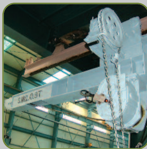
Fuel Oil Hose Handling Davit (Mono Rail Type)
